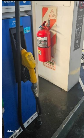
Extintor PQS 7kg
